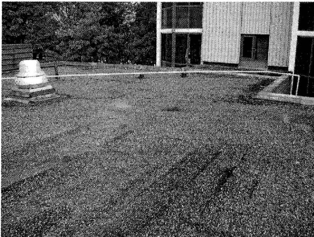
Picture 2: Ridges and boils in tar and gravel roof.
