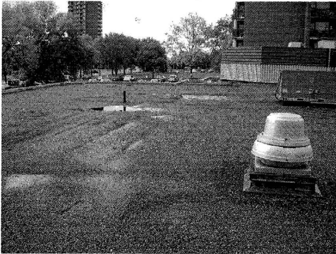
Picture 3: Water ponding and patches in area of leaks shown in Picture 1.
